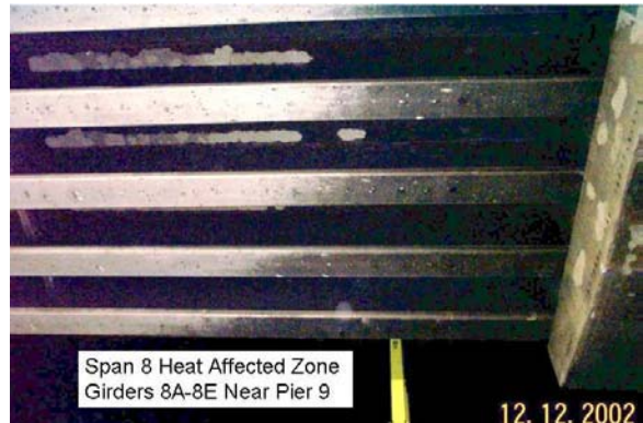
Photo 2. Span 8 Heat Damaged Flanges
