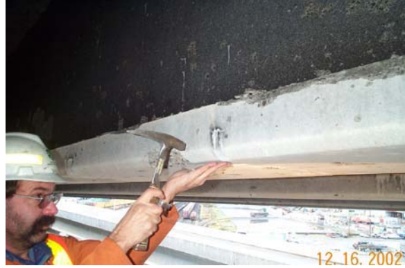
Photo 4. Crumbling Concrete Girder 8E
